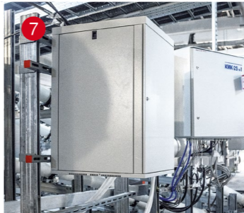
Equipment supports and platforms
