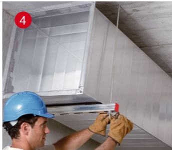
Mechanical & Electrical, HVAC
