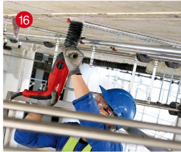
Post installed anchors
