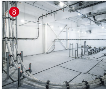
High voltage cabling supports
