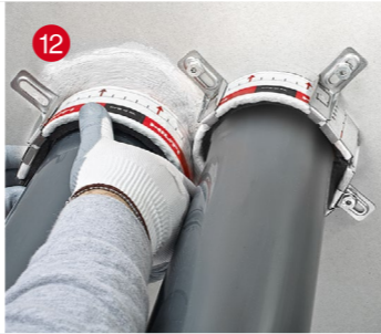
Piping and ventilation
